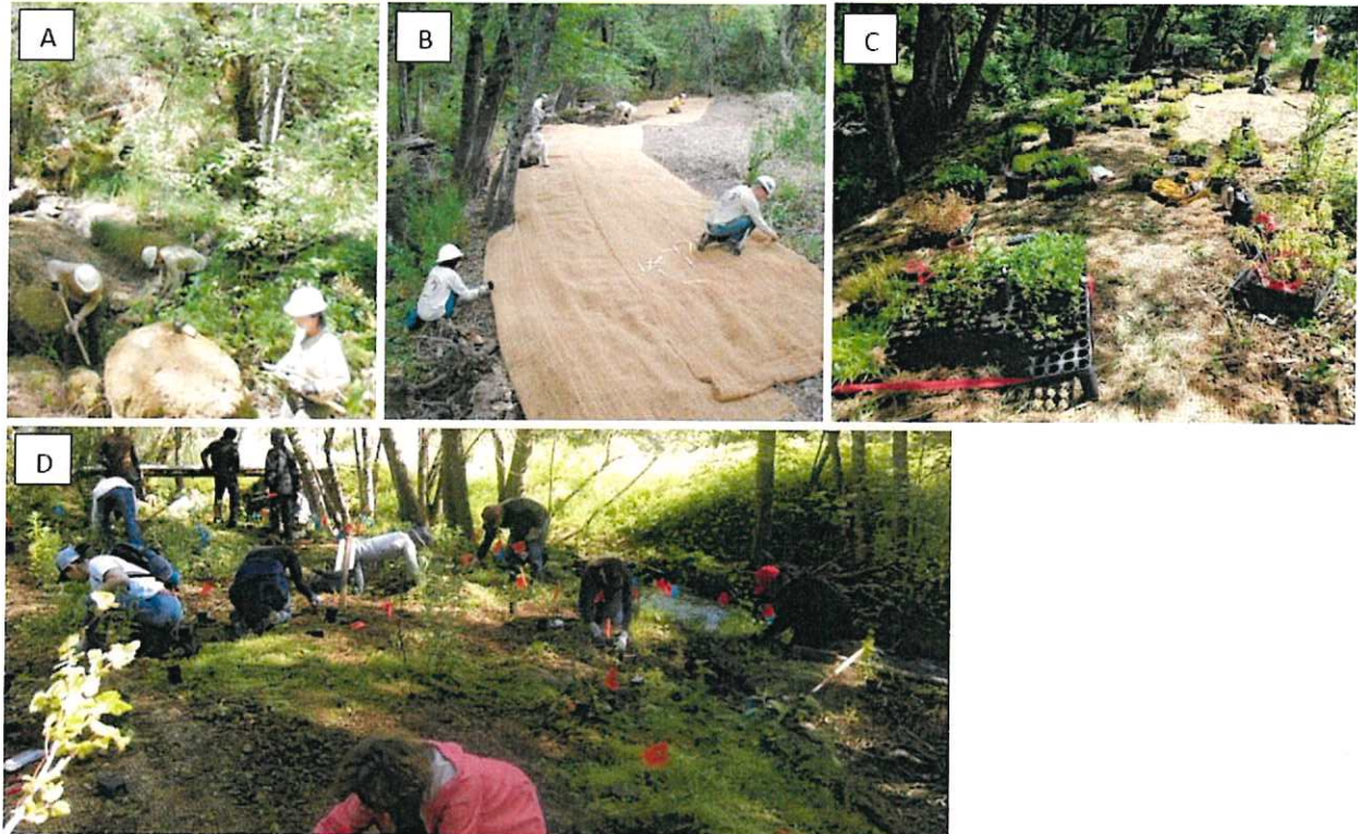
Figure 1. (A) American Conservation Experience (ACE) crew removes invasive species within the LTNC's Conn Creek riparian project area on the Linda Falls Preserve. (B) ACE crew installs erosion control blanket along Conn Creek after removing invasive Himalayan blackberry, which dominated the site. (C) Native plants, propagated from material collected within the project area, staged for planting in previously invaded areas. (D) Land Trust volunteers plant native species in a previously invaded site.
